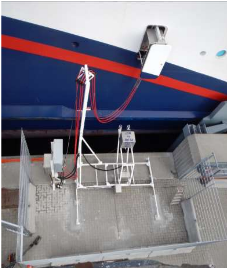
PLUG automated mooring system on Color Line Superspeed 2 at Larvik
